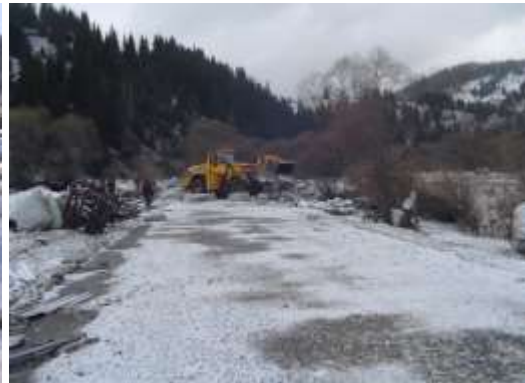
Fig.6 C. Evacuation of ice packs reaching DN 17B national road, Suceava County (photo Gavril Petrică)
