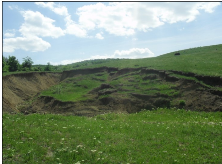
Fig. 4. Collapse of the sliding cornice
