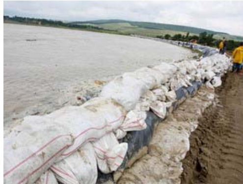
Fig. 7 - Dam of Rogojeni, Galati County, on the lower Prut - 15 VIII. 2008 (ISU Galați)
