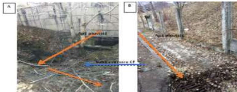
Fig. 3. Drainage channel A: in the right side of the ramp (drain pipe and chimney) and B: in the left side of the ramp, after undercrossing CF (chimney and collector ditch)
