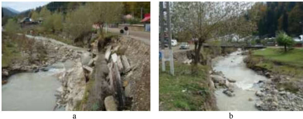
Fig. 4. General view of the morphology of the Tazlăul Sărat riverbed and the state of degradation of shore defence and DC 180A in Zone 1 "Toderaş": a - general view from downstream with highlighting the erosion of the road; b - upstream view (Oct 2016)
