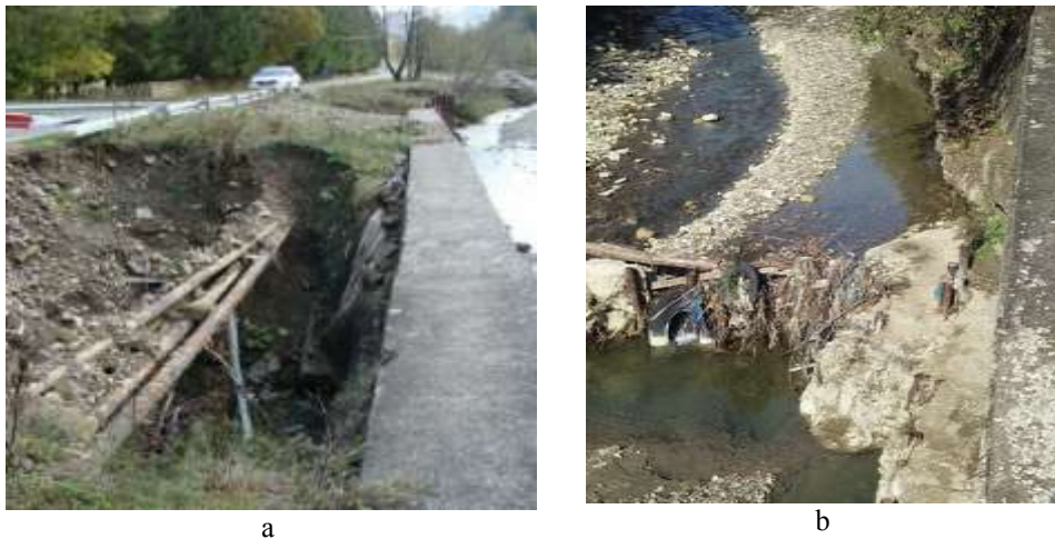
Fig. 7. Erosion phenomenon of the left bank after the flood in June 2016 on the Tazlăul Sărat River in Zone 4 "Forest Canton of Maxim": a - general view of the erosion zone behind the shore defence at the DC 180A limit; b - fencing phenomenon in the shore defence foundation area (Oct. 2016)
