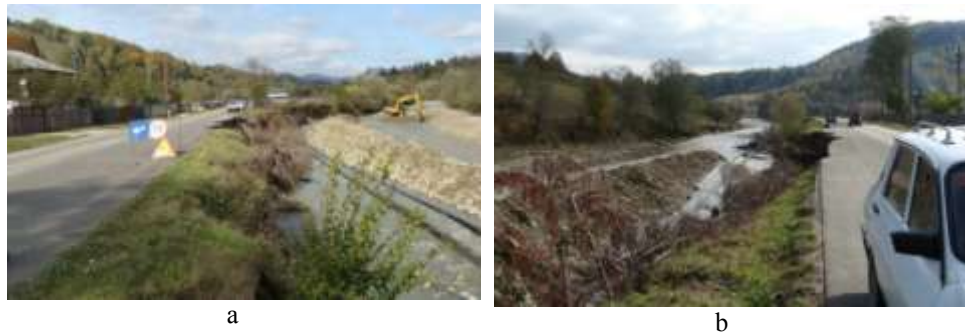
Fig. 5. The degradation phenomena of the riverbed in Zone 3, "Chiosa" after the flood in June 2016 on the Tazlăul Sărat River: a - upstream view of the river bed change and erosion; b - downstream view, highlighting oil piping and breaking the DC180A (photo Oct 2016)
